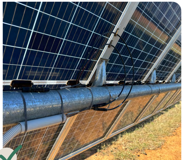
Wires inaccessible to sheep
