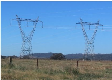
Tall and wide steel lattice
