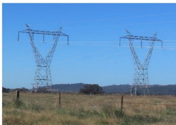
Tall and wide steel lattice
