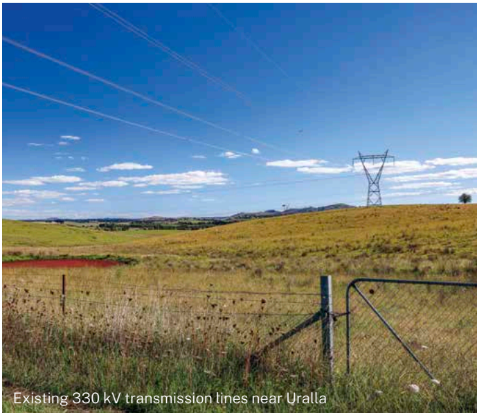
Existing 330 kV transmission lines near Timbumburi
